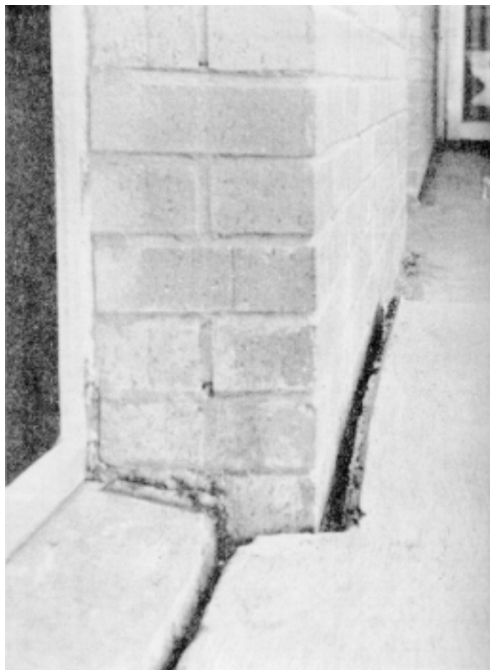
Figure 32. —Damage to foundation of church built on Houston Black clay. This building is less than 2 years old.
